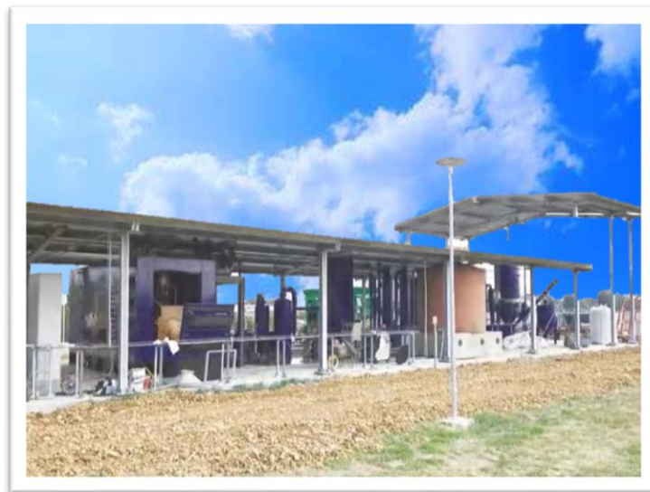
Italy (Venice) H2life plant - 200KWh
